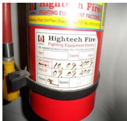
(a) Expired fire extinguisher
