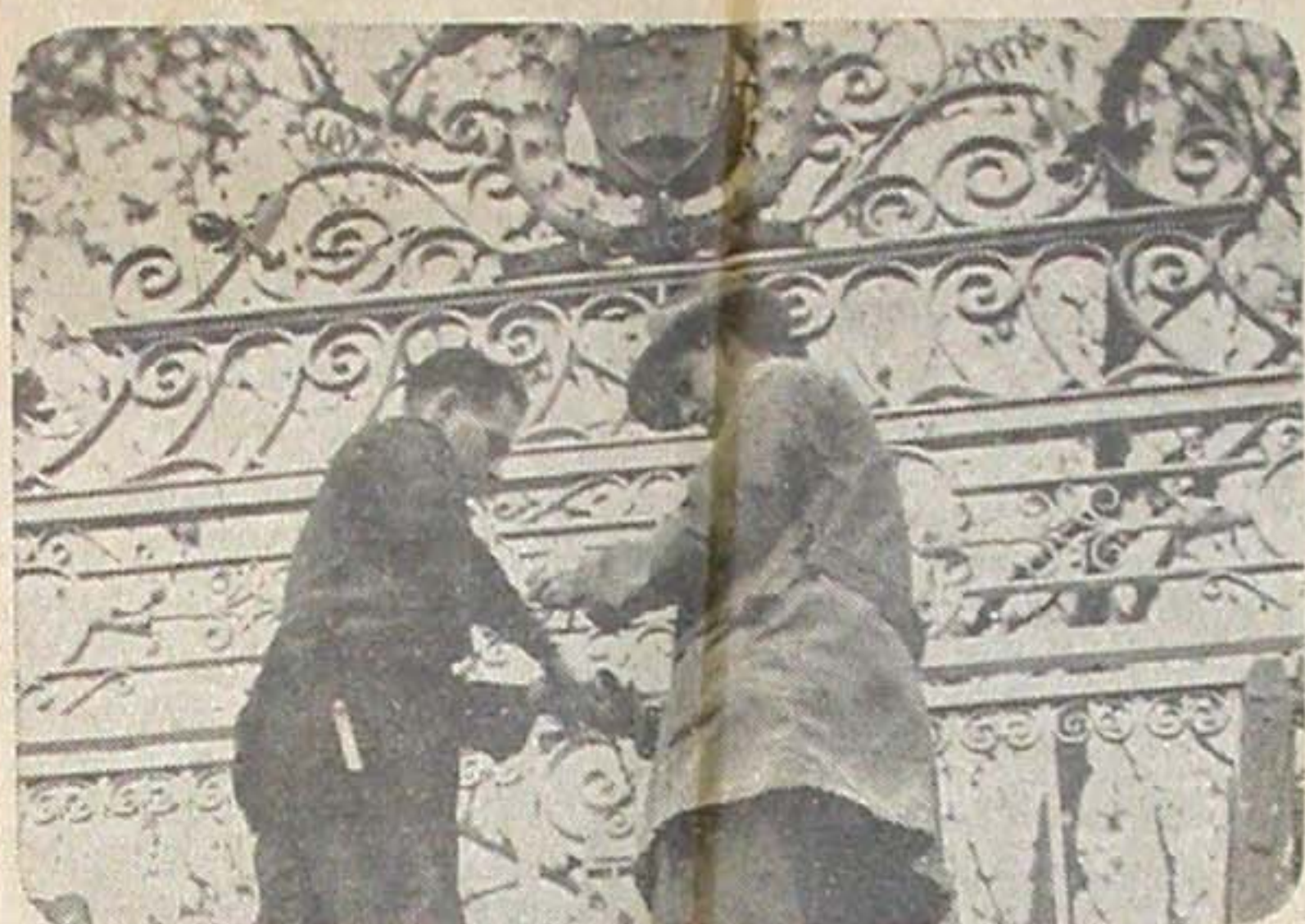
WORKMEN PUTTING FINISHING touches to the new big entrance gates to the Jubilee Oval and Barr Smith Library today.
