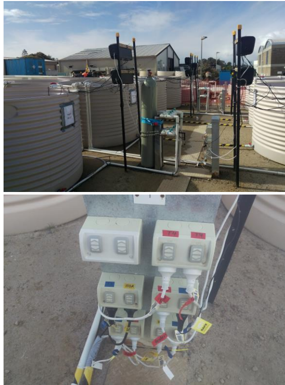
Figure 3: Top: The electrical power boards can be seen in the middle of the image, attached to star droppers and plugged into outdoor electrical outlets. Bottom: The colour coded electrical outlets for easy on/off procedures.
