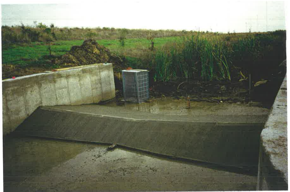
Photograph 4.17 The completed Henschke Street weir (drain is dewatered). The steel mesh cage is not shown in the correct position.
