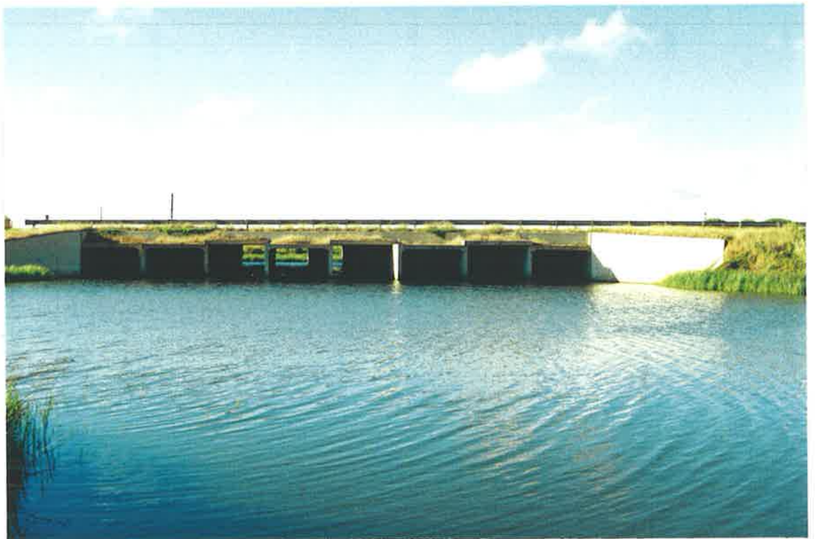
Photograph 5.10 Culverts taking water from the outlet of Pond 4 underneath South Road Connector/Salisbury Highway. (Photograph taken facing North)
