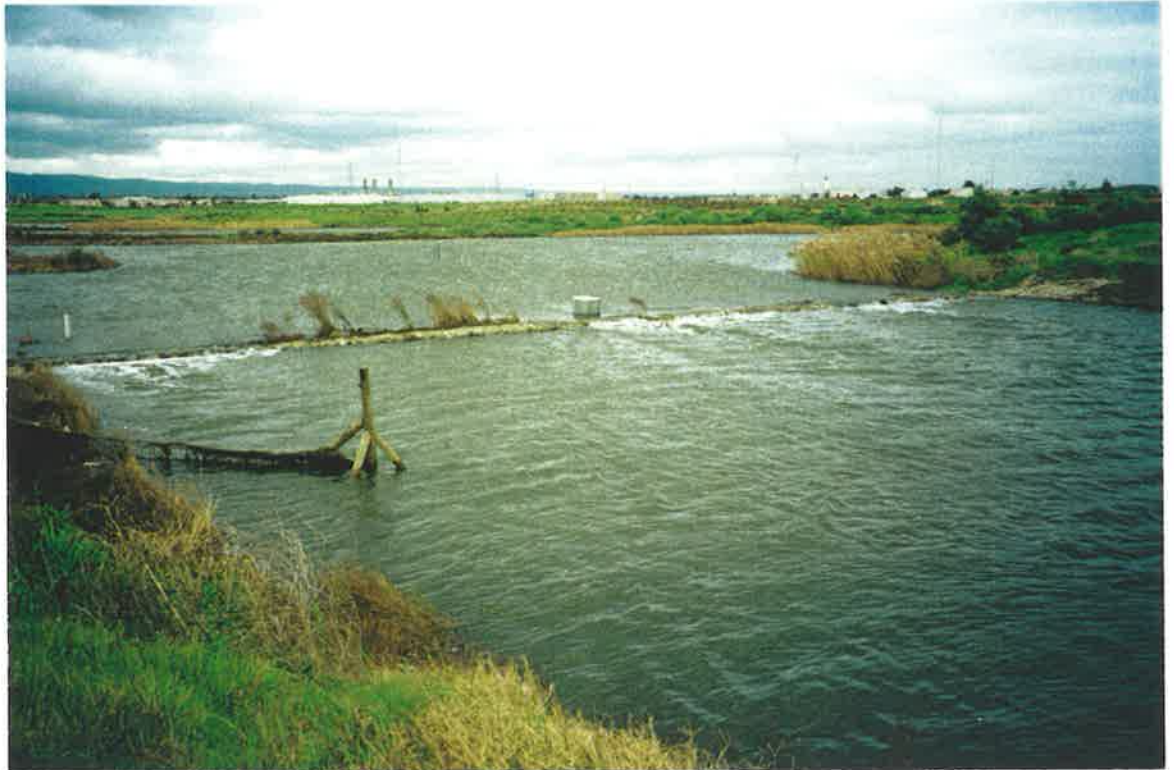
Photograph 5.11 Flow over rock gabions which are beginning to act as a broad crested weir
