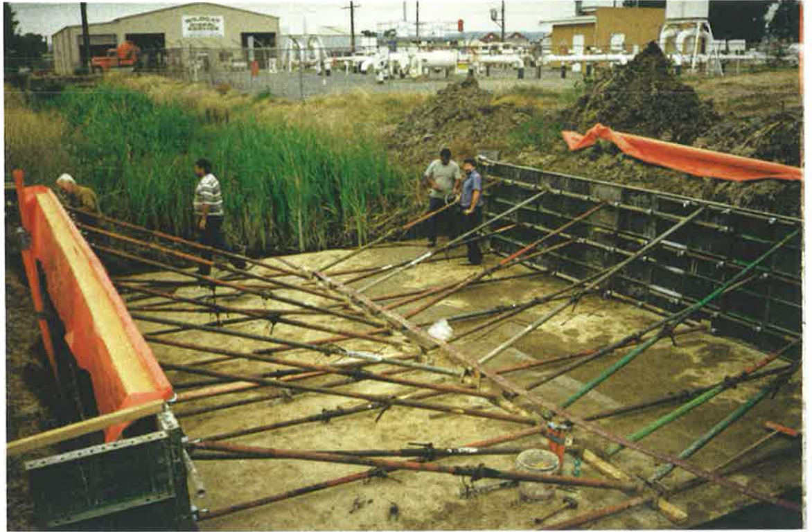
Photograph 4.16 Henschke Street monitoring station during construction.
