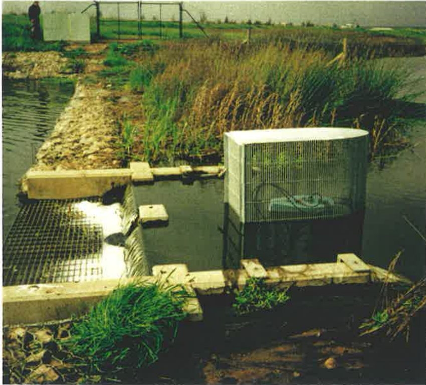
Photograph 5.9 Outlet structure at the South Road Connector station which the shows sharp crested weir and rock gabions either side.
