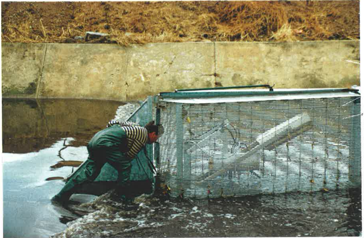
Photograph 5.1 Instrumentation cage at North Arm East containing water quality probes.
