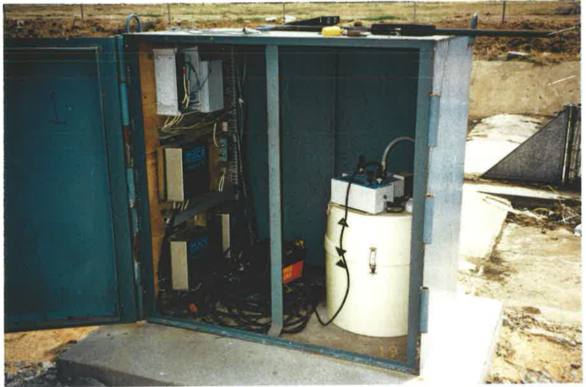
Photograph 5.3 Instrumentation cabinet at North Arm East containing data logger and controller, battery power supply, and automatic water sampler on the right.
