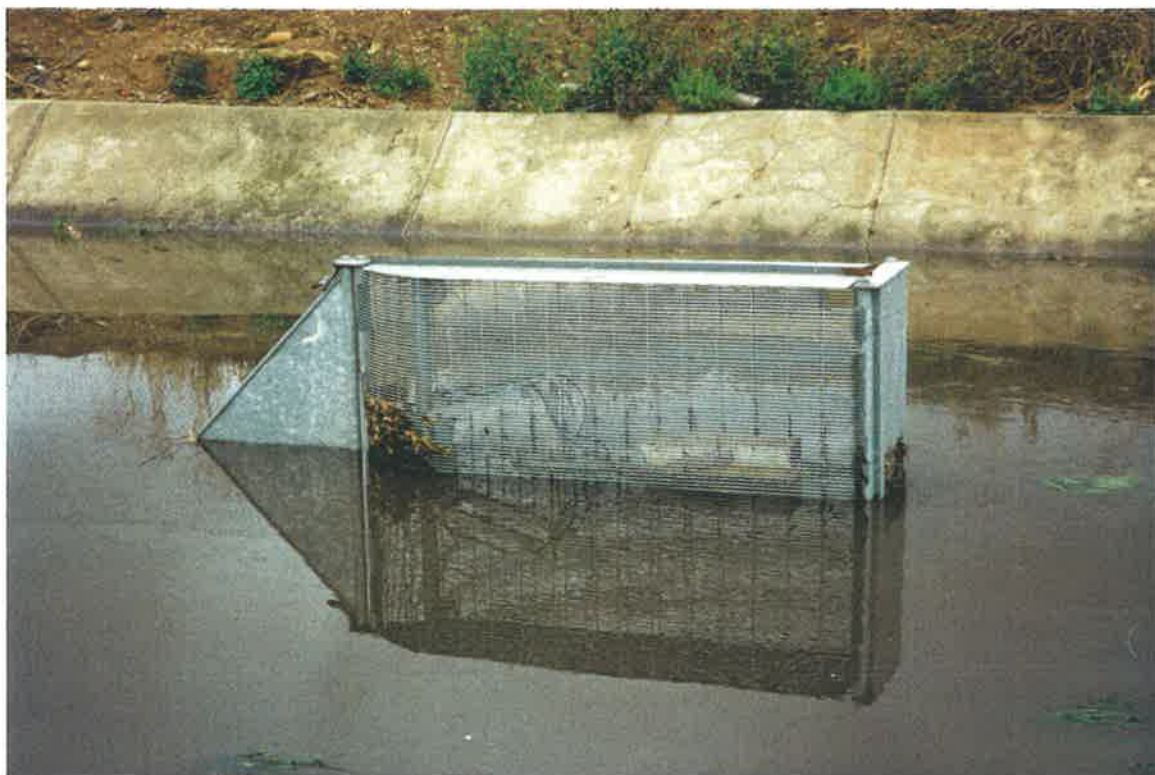
Photograph 5.8 North Arm East weir during an event after the installation of the trashracks. Note there is NO drop over the weir, which is completely drowned out.
