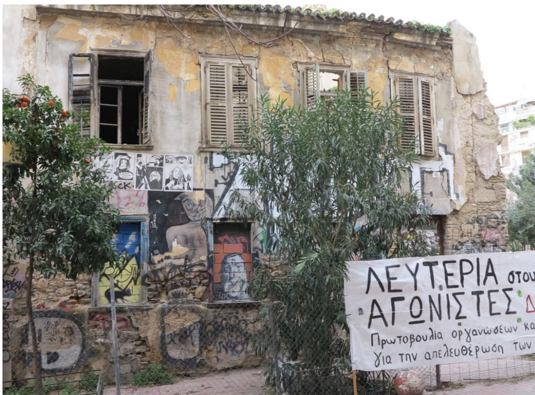
Figure 4.7 Derelict neoclassical house in Exarchia
