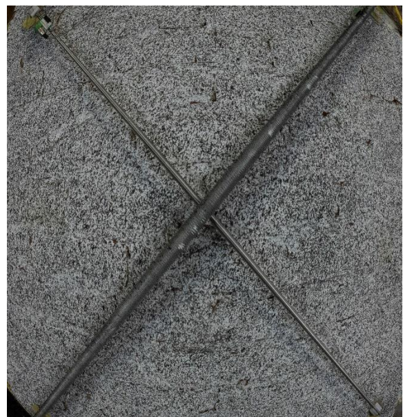
(b) distorted masonry panel image
