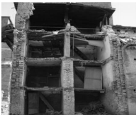
(a) wall collapse under out-of-plane load
