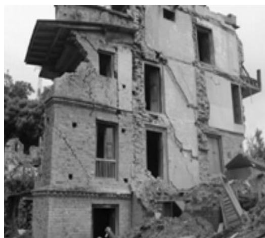
(b) wall failure under in-plane load
