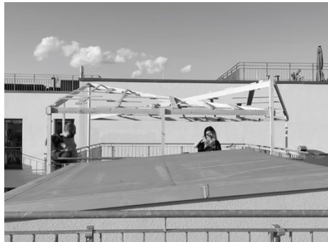
Fig. 94 | Architectural adjustments can provide a sense of completion to external spaces. How often are such actions avoided due to forces of the public gaze?
