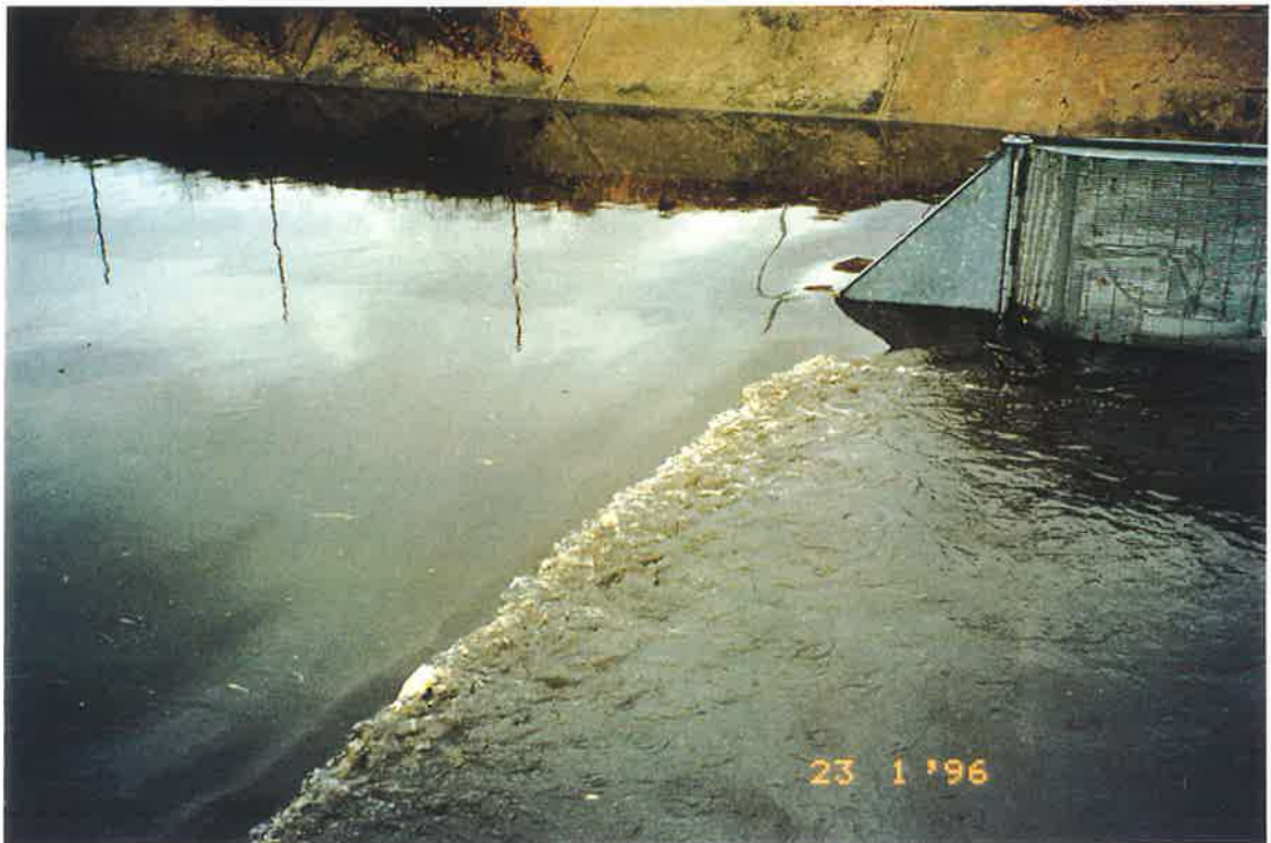
Photograph 5.3 : Storm event prior to the installation of trash racks. No backwater
