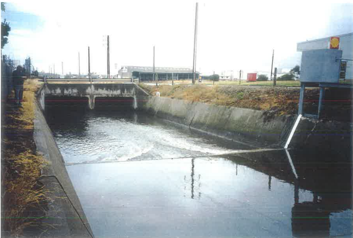
Photograph 3.24 : The Monitoring station at the Eastern Parade Drain (AU504201). Facing Downstream.
