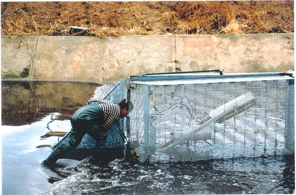
Photograph 4.4 : Instrumentation cage in the North Arm East Drain
