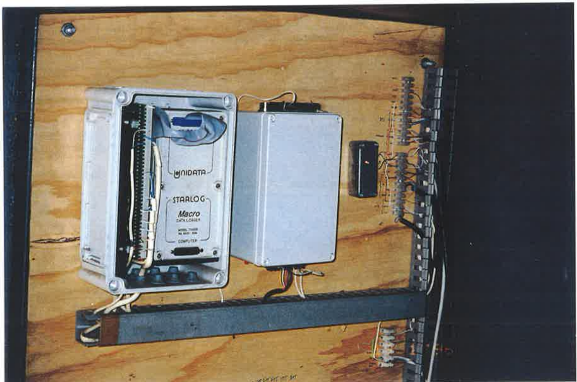
Photograph 4.7 : Data logger and controller.
