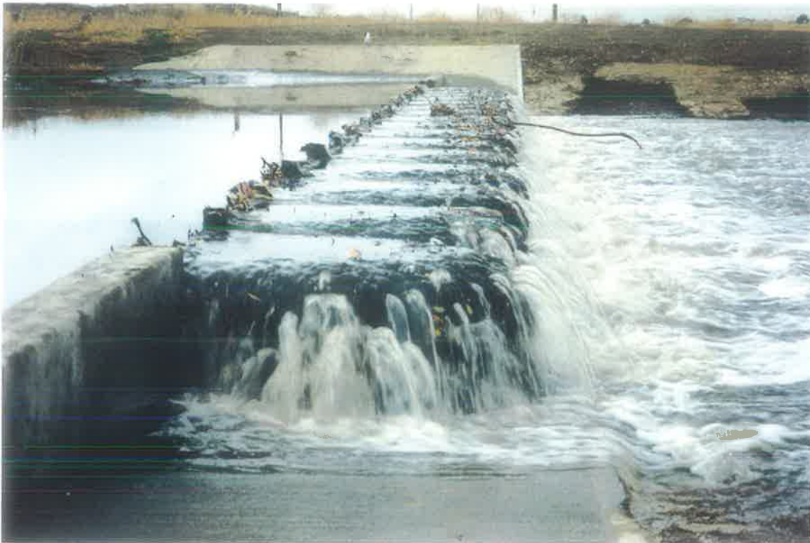
Photograph 5.1 : Trash racks in the North Arm East Drain
