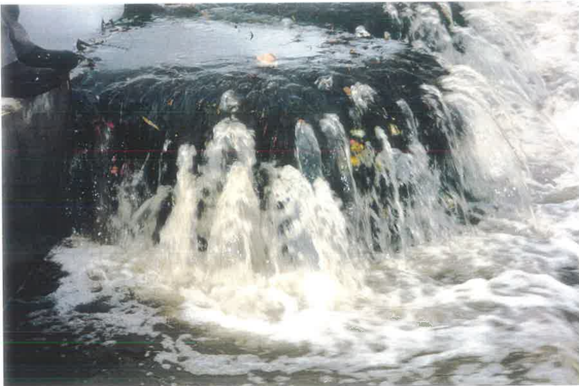
Photograph 5.2 : Trash rack basket full of gross pollutants
