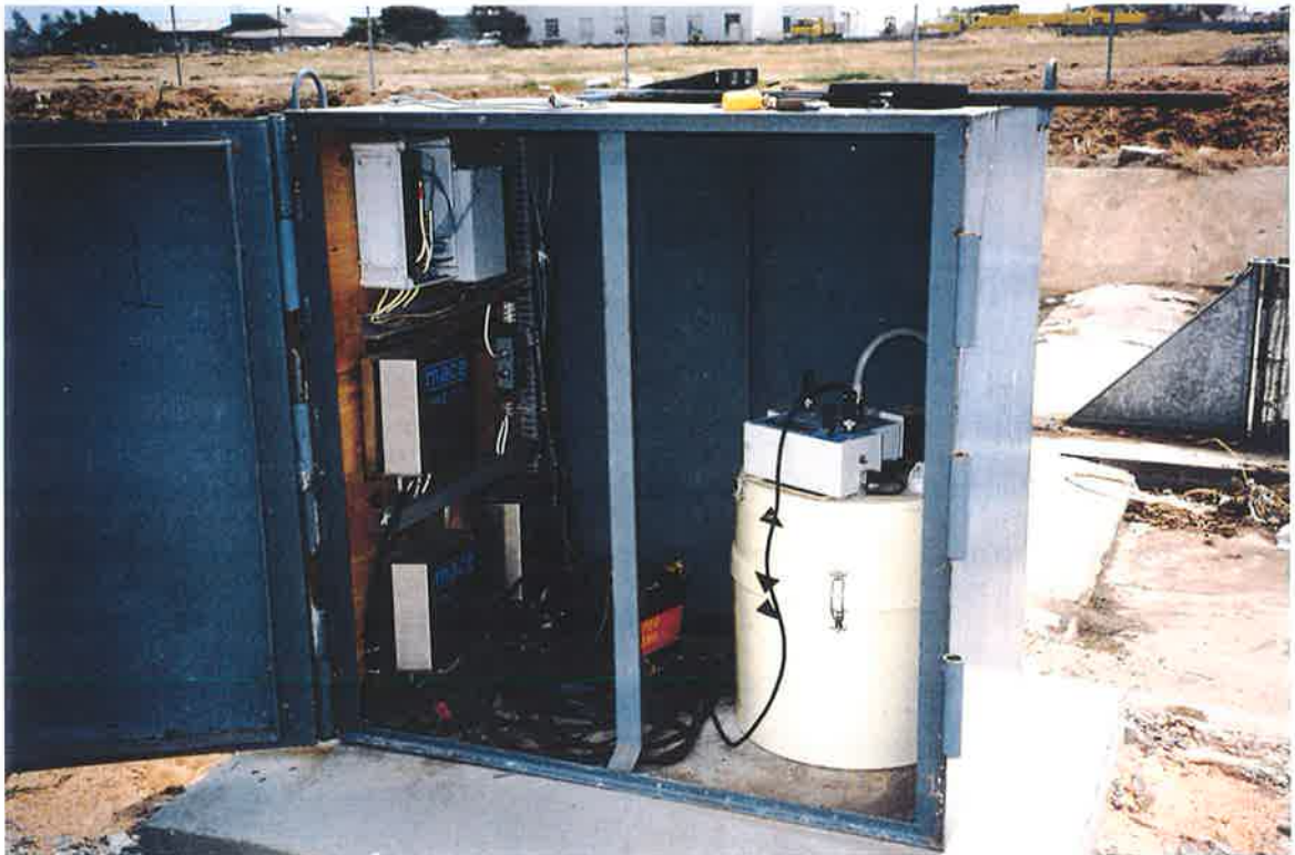
Photograph 4.6 : Instrumentation cabinet at the North Arm East Drain.
