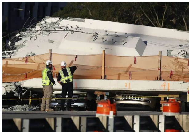
Figure 1.1 Collapse of pedestrian bridge [1]
