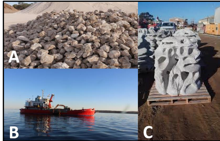
Fig. 1. Construction of Windara Reef in 2017, showing A) the limestone boulders used to construct the reef, B) construction vessel MPV Andrew Wilson constructing the reef and C) a custom-designed concrete structure used to construct the reefs. Images taken by: Department of Primary Industries and Regions, the Government of South Australia, 'Shellfish reef construction', sourced on 25 th of January 2022, https://www.pir.sa.gov.au/fishing/recreational_fishing/windara_reef/shellfish_reef_construction
