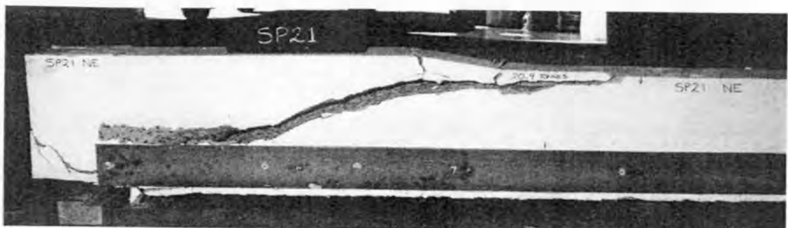
(b) Failure of SP21
