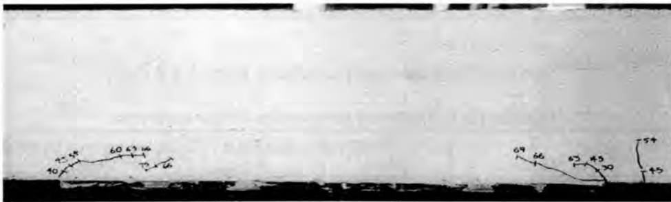
Fig.12.5. FP-T20: Crack pattern near plate ends at debonding
