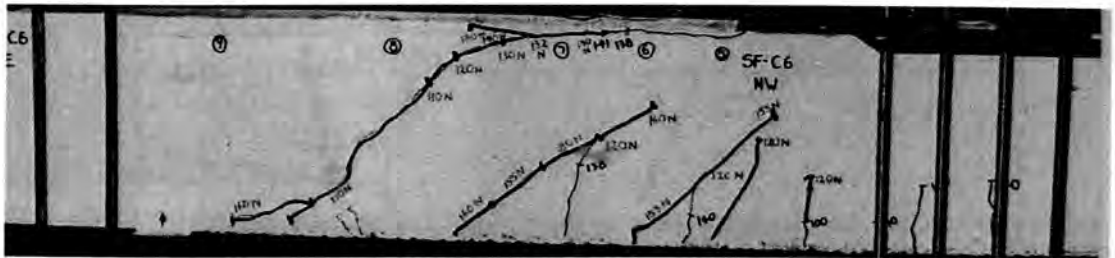
(a) Crack pattern on north side
