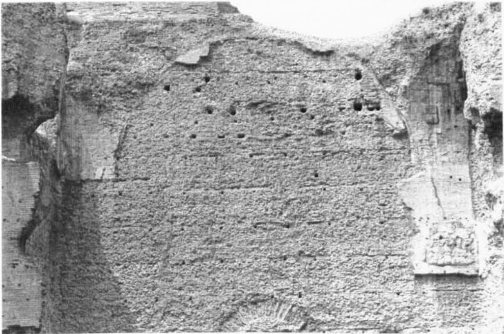
Fig. 65: Baths of Caracalla, central block, Rm 4E, W wall, bonding courses and putlog holes.
