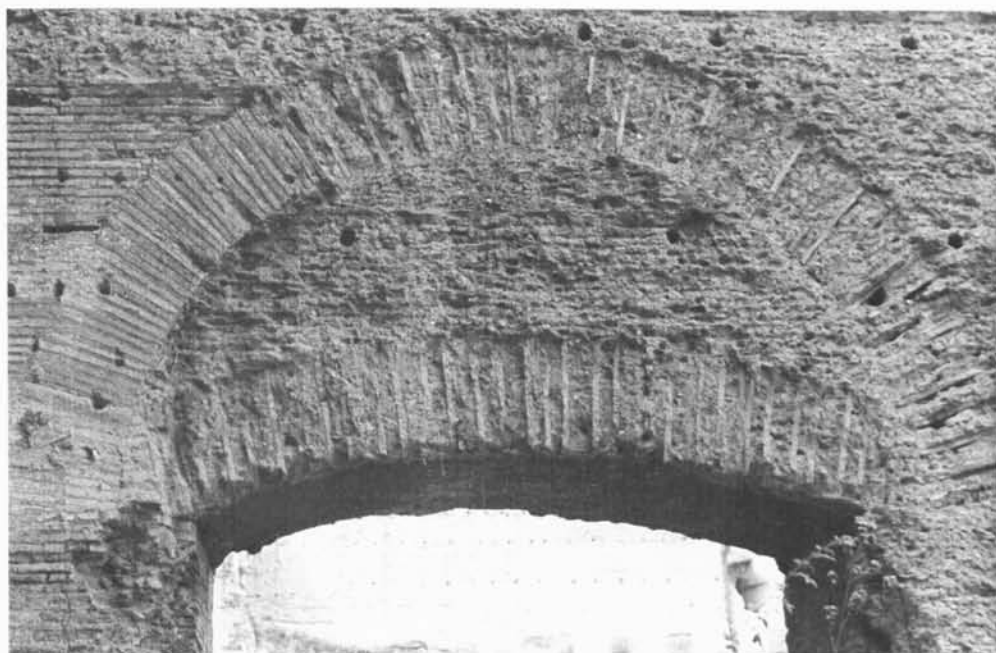
Fig. 72: Baths of Caracalla, central block, Rm 4W, detail of arch construction over door to Rm 12W.
