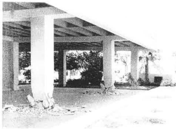
Fig. 1.2 Typical flexural plastic hinge failure of columns (Green, 1987)
