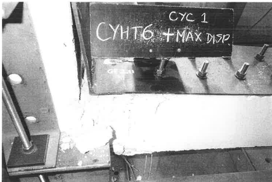
Fig. B.72 Front view at -100mm displacement for specimen 2BCP6G
