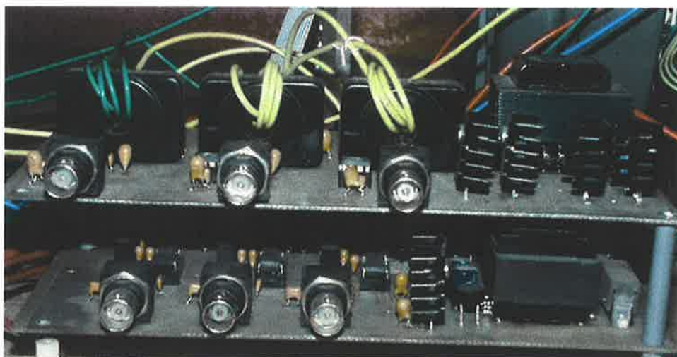
Photo D.3 Current and voltage transducers
