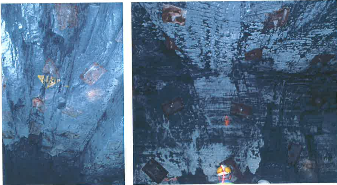
Figure 4.19. Joint swarms observed in the underground workings. The figure on the left is of the roof. The steel plates are about 300 mm long. The joint swarms extend the full height of the underground adit (4 m) and occur in zones 2–20 m wide. Joint spacing is in the range 50–500 mm and joints were only observed in the coal.
