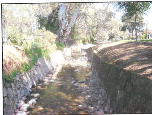
Figure 8.2. Open-engineered study reach in Third Creek. The channel straightening, consistent width and flat concrete base is evident. The rocks embedded in the base trap gravel and generate some spatial heterogeneity.
