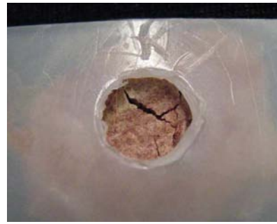
(b) Cracks visible on the underside of the same sample
