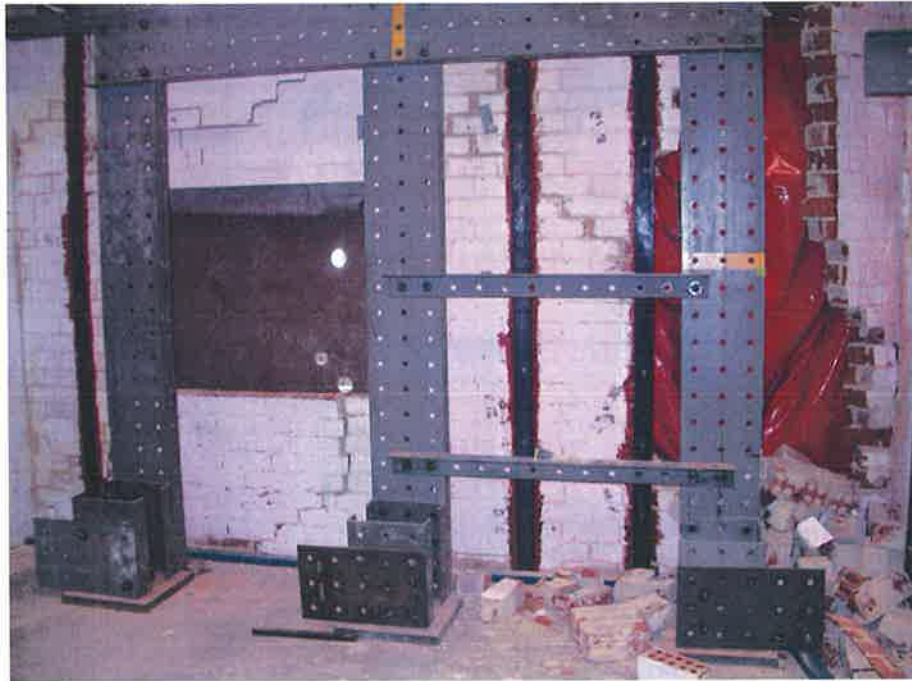
(a) Overall view of failed Wall 3
