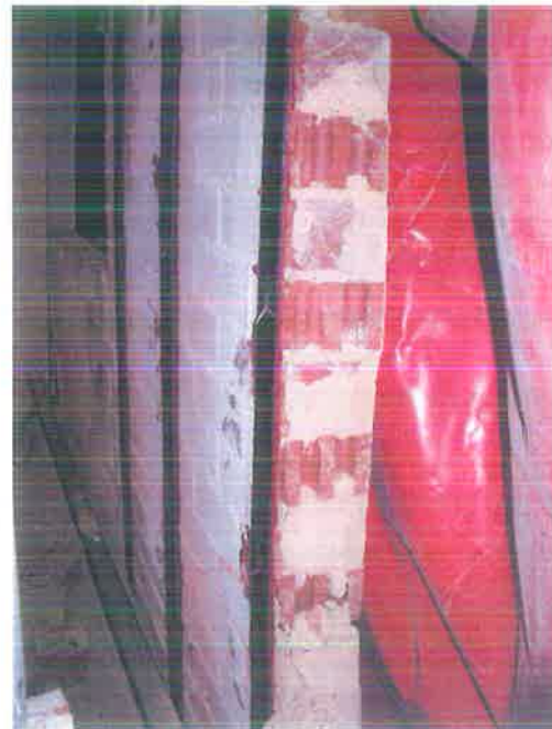
Masonry failure surface
