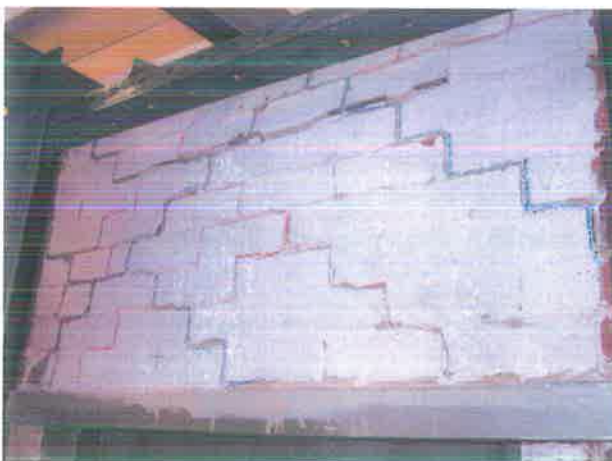
Cracking above the window
