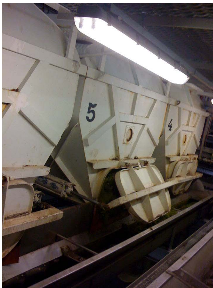
Figure 7.13: Miller static drainers (door of drainer #5 opening to evacuate pomace onto screw-conveyors)
