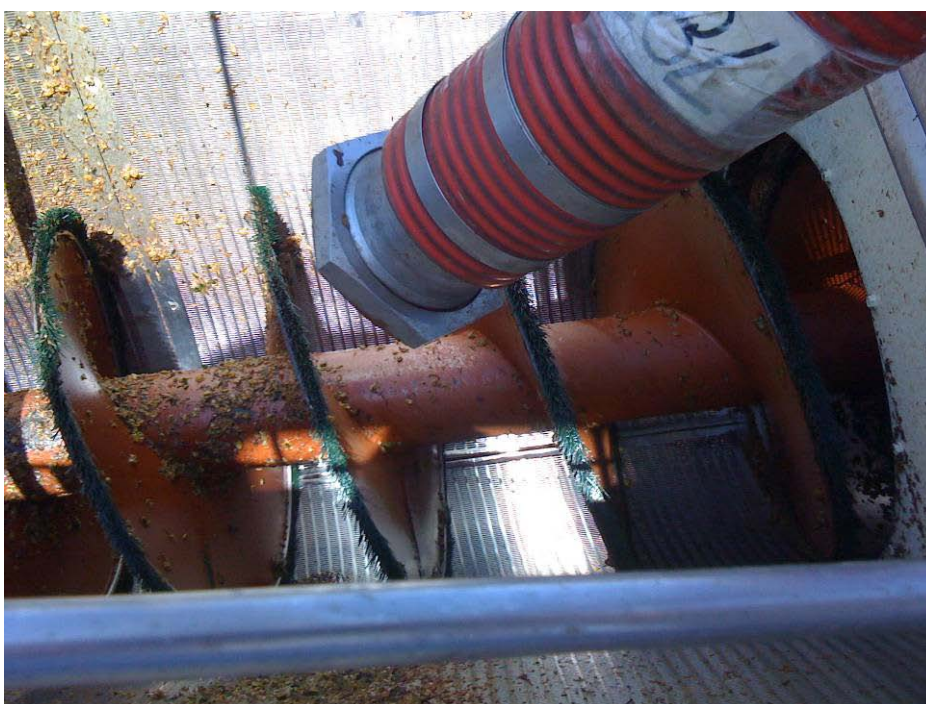
Figure 4.13: Inclined drainer feed hopper with brushes on screw thread
