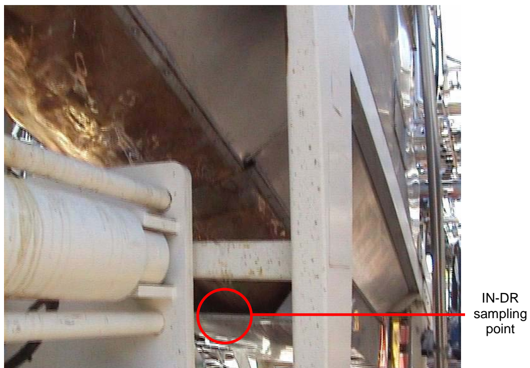
Figure 7.10: Underside view of inclined drainer (sampling location marked)
