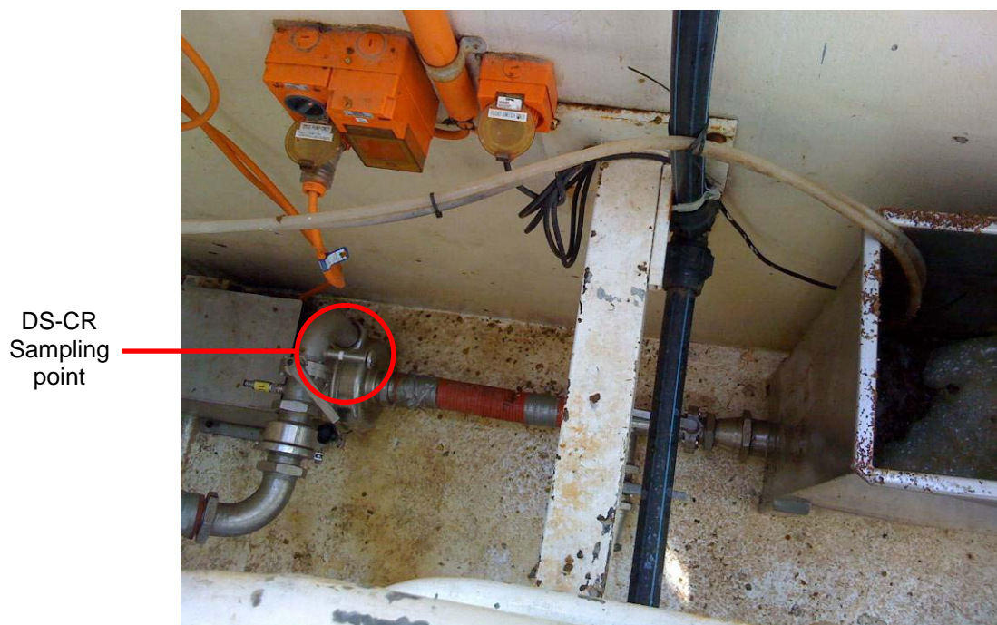
Figure 7.7: Centrifugal pump for pumping out destemmer-crusher run-off buffer (sampling location marked)
